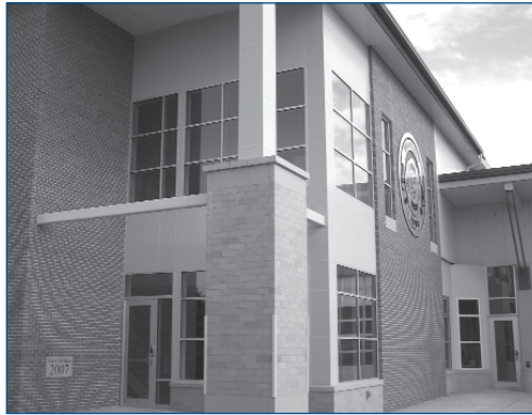
A view of the front entrance. Just left of the fire department logo is the intersection of the conventional steel structure and pre-engineered steel structure.
